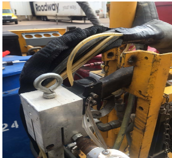
Nylon Protective Hose Material Secured From Dispensing Valve Continuous Into Chemical Hose Bundle
